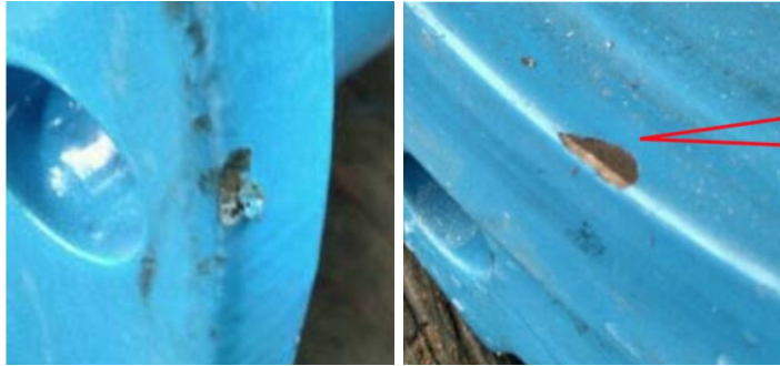
On DN200 Gate Valve
